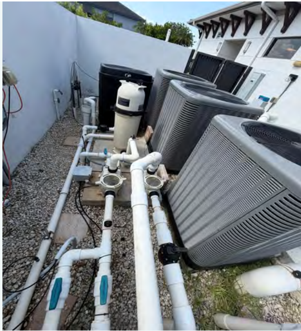
Figure 1. Multiple heating and circulation components in a constrained equipment area.
