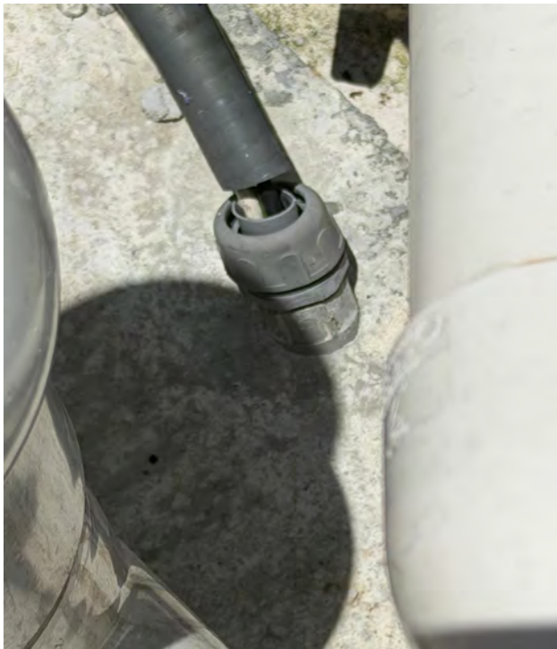
Figure 3. Visible separated flexible raceway/connector condition requiring evaluation by the responsible licensed electrical professional.
