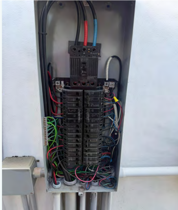
Figure 2. Existing electrical panel serving numerous circuits and large connected loads; full circuit tracing and load verification are required.
